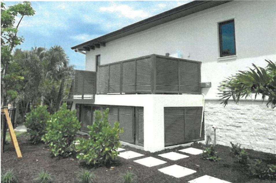
(06/11/2026) Elevated AC & Generator Platform, Kayak Storage Below
