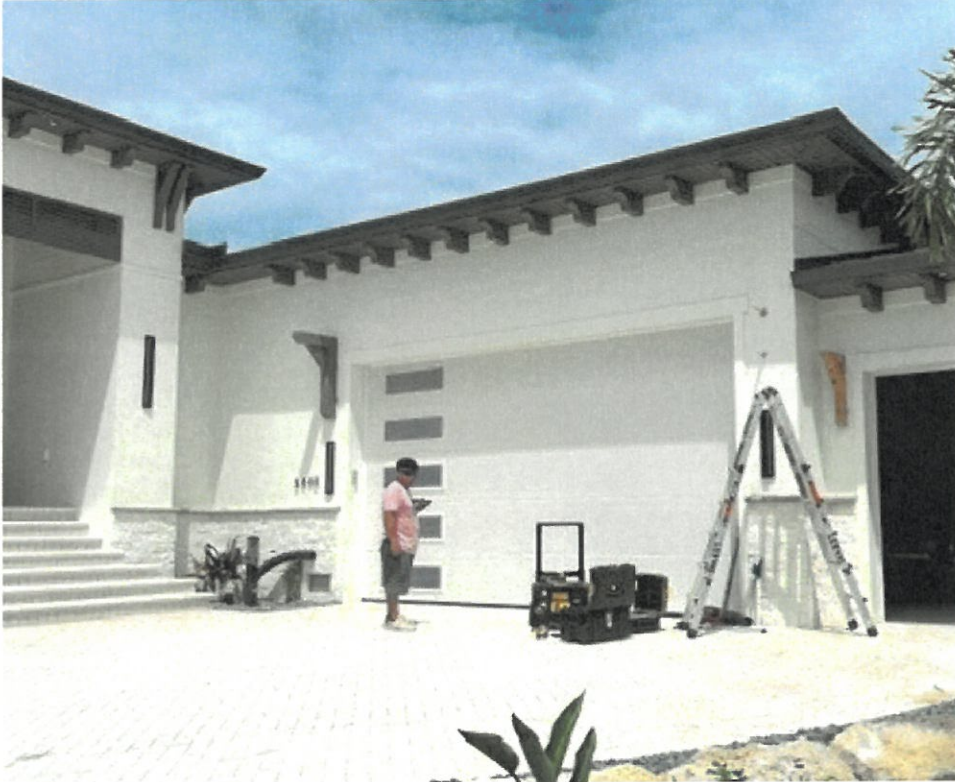
(06/11/2026) 1 Smart Vent in Face of Garage Wall at Steps
