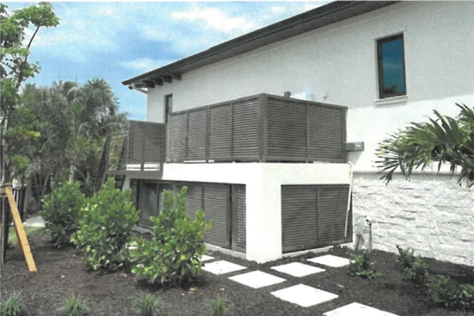
(06/11/2026) Elevated AC & Generator Platform, Kayak Storage Below
