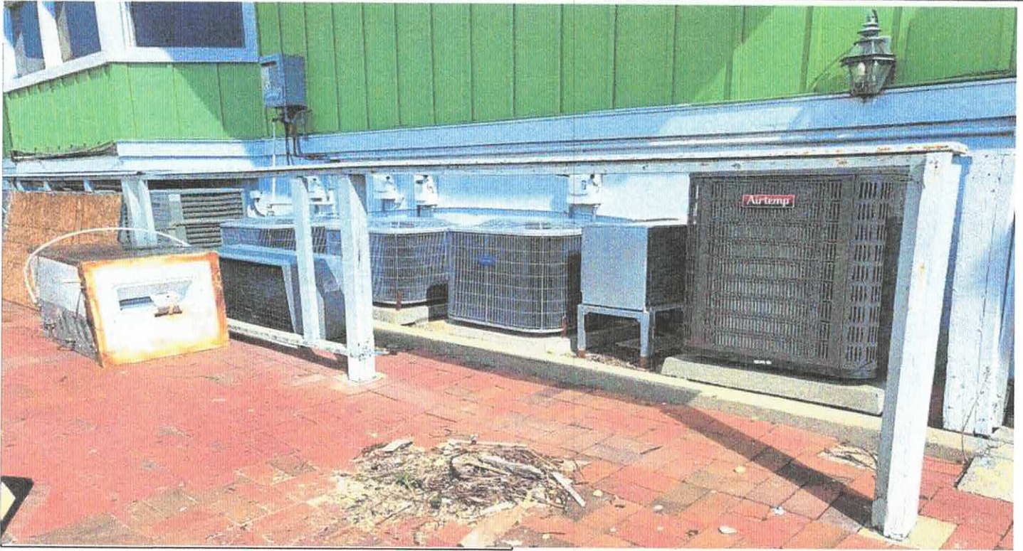
AIR CONDITIONER PHOTO TAKEN ON AUGUST 18, 2025
