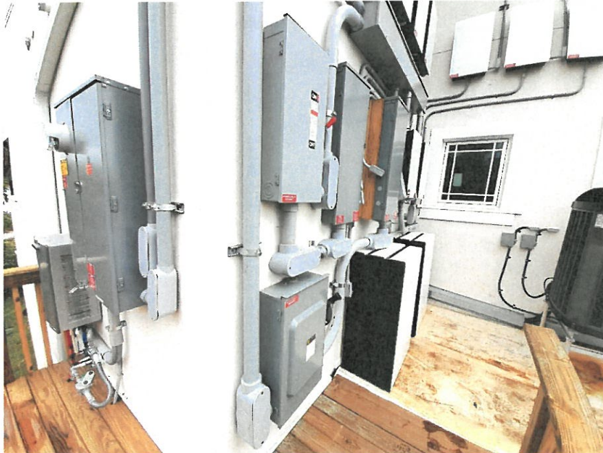
(06/13/2024) Raised Equipment Platform. Lowest Equipment= Tankless Water Heater next to Electric Meter Box= 22.6'. AC Units= 22.8'
