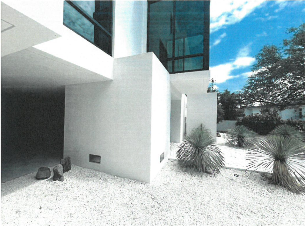
(04/18/2024) 2 Smart Vents in Storage Area Walls
