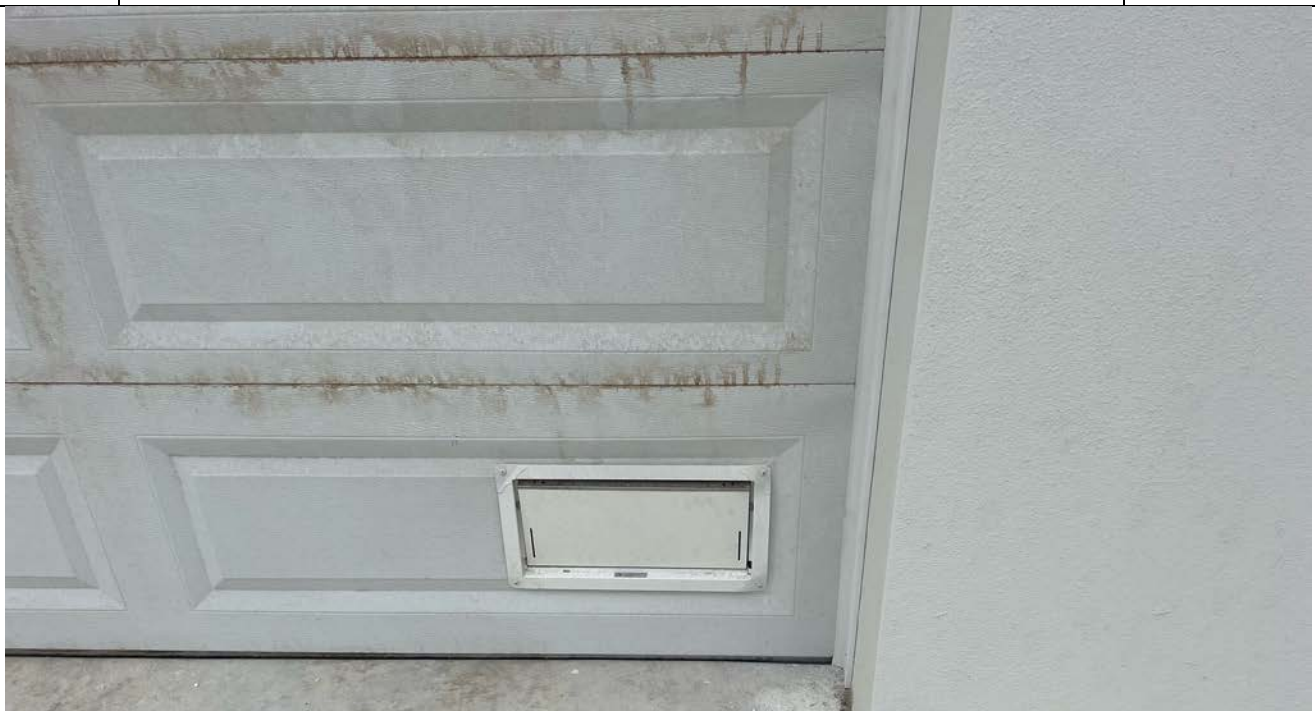
Photo 6 Caption Smart Vent Detail JOB# 20-1466 Date Taken 5/15/23
