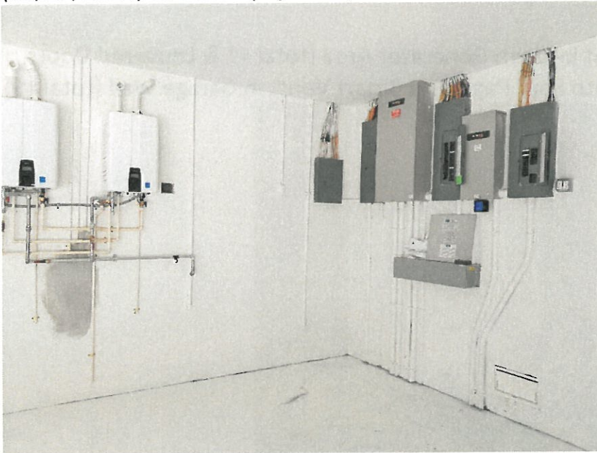
(06/17/2024) Lowest Equipment, Water Heaters on Wall Inside Garage
