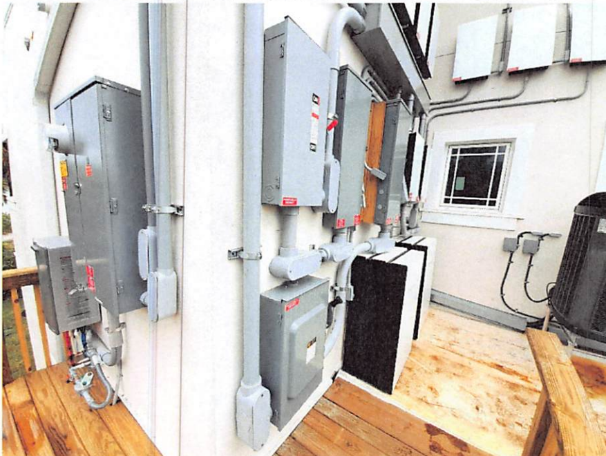
(06/13/2024) Raised Equipment Platform. Lowest Equipment= Tankless Water Heater next to Electric Meter Box= 22.6'. AC Units= 22.8'
