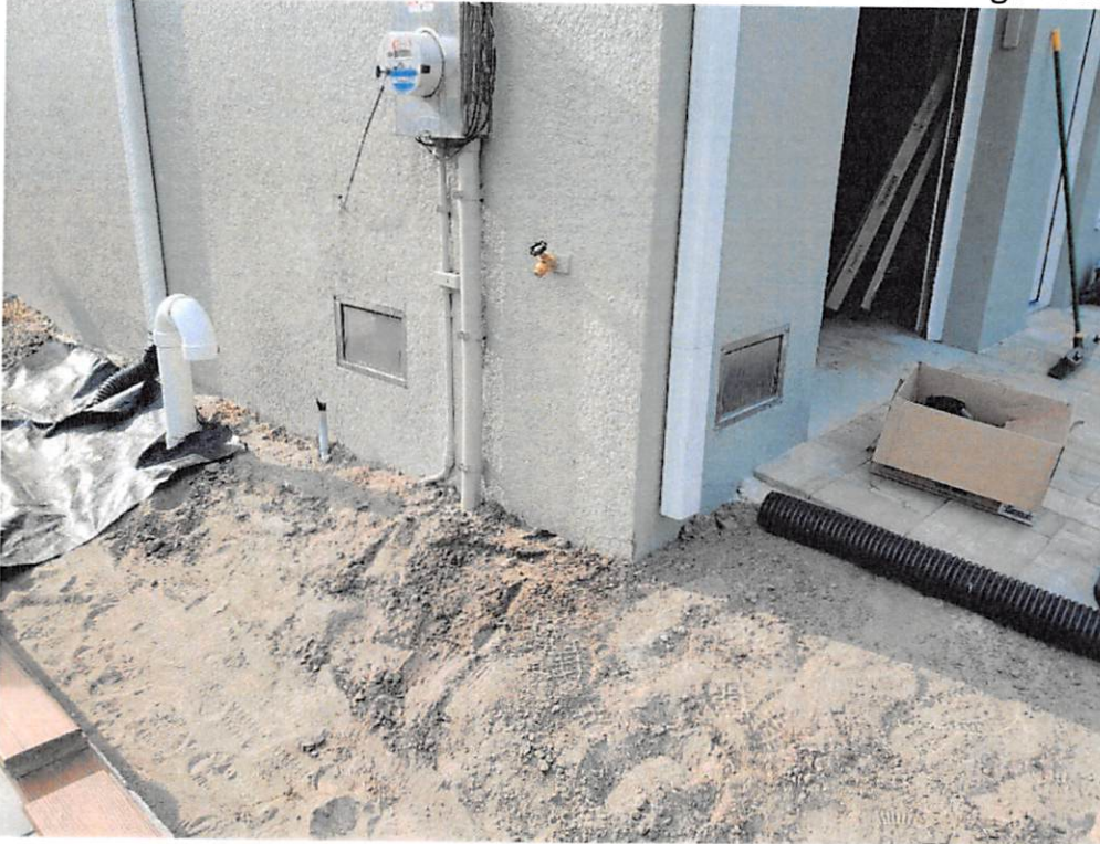
(05/31/2023) Typical Smart Vent Model #1540-570 in Garage Walls
