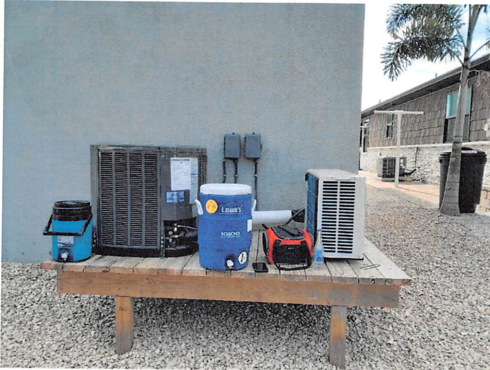
(05/31/2023) Elevated AC on Platform on Rear of House
