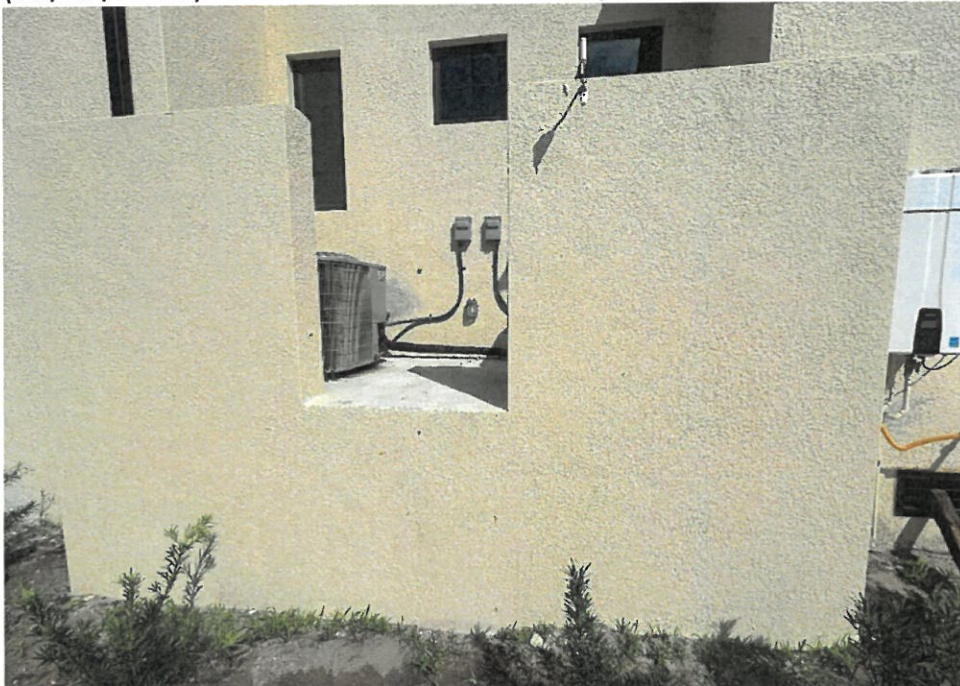
(05/27/2025) Elevated AC Enclosure Top of Slab=11.1'
