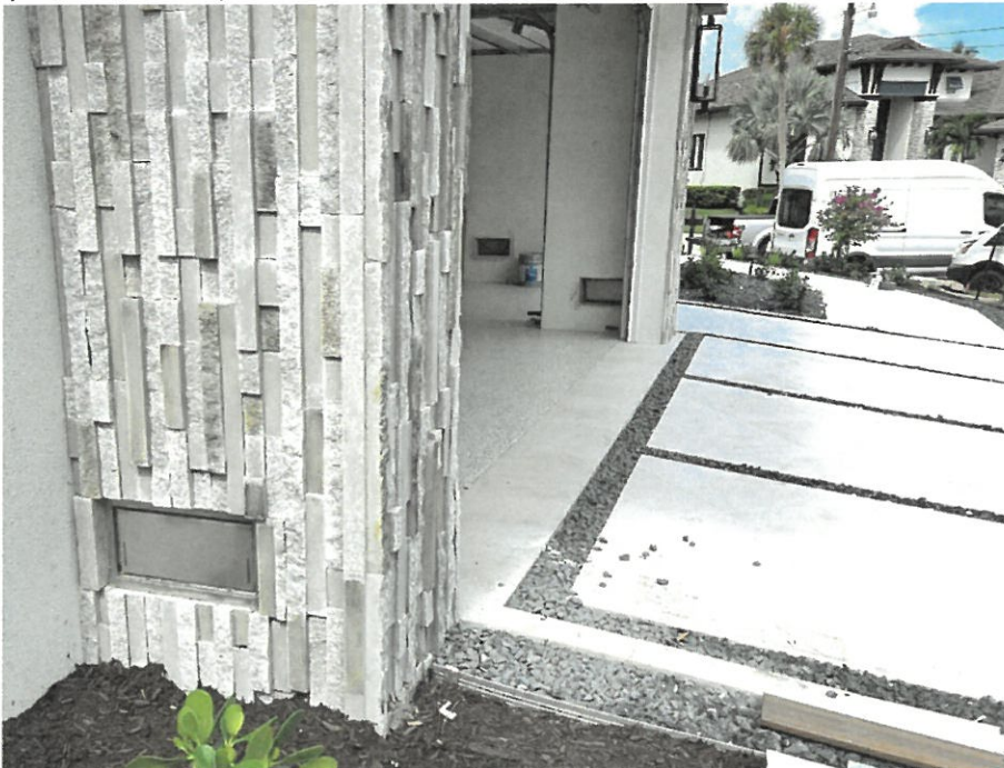
(08/13/2025) 2 Smart Vents Model #1540-520 on Front Wall of Garages
