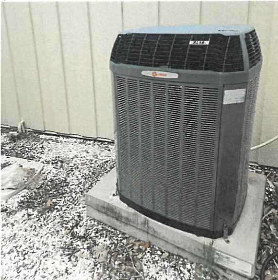
(07/01/2025) AC Unit on Slab Outside of House
