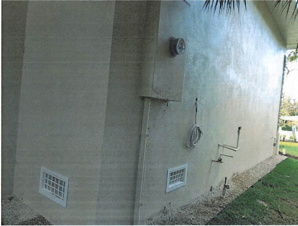
(11/08/2023) Typical Flood Flap Model #FFWF08 in 2 Car Garage Walls (3 Total)
