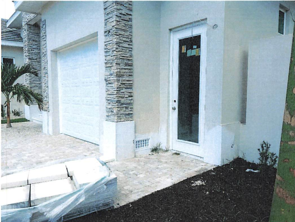
(11/08/2023) Typical Flood Flap Model #FFWF08 in 1 Car Garage Walls (2 Total)
