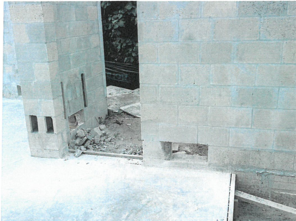
(02/20/2023) 2 Flood Openings in Back Walls of Garage/Entry area
