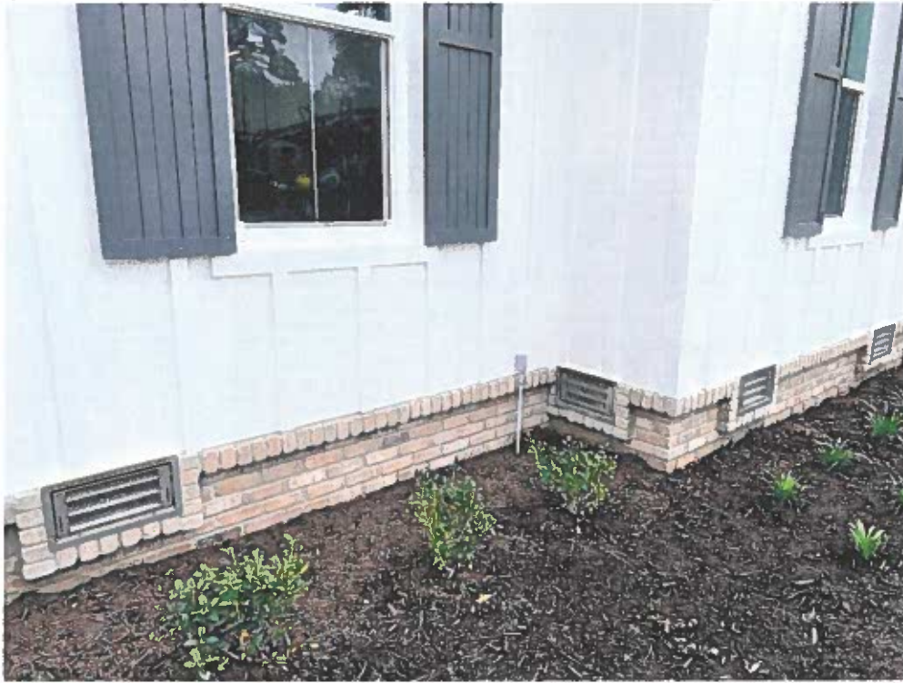
(03/03/2023) 4 Smart Vent Model #1540-510 on Right Side Garage Wall
