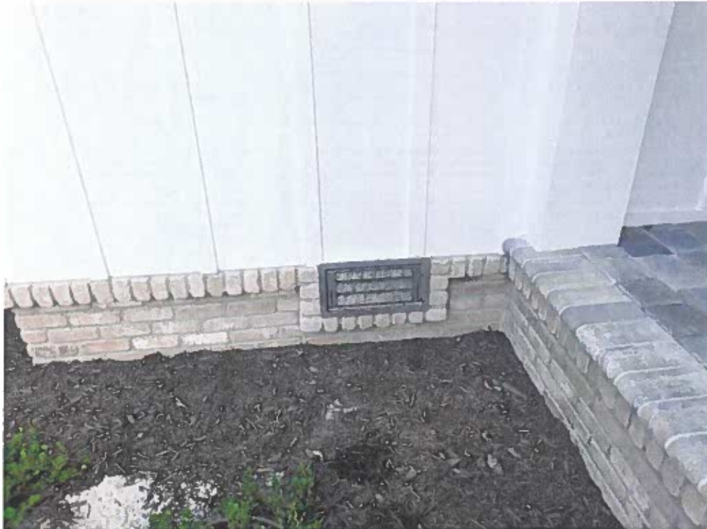
(03/03/2023) 1 Smart Vent Model #1540-510 on Front Garage Wall
