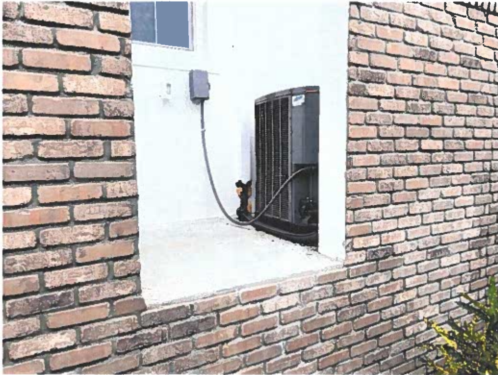
(03/03/2023) Elevated AC Unit in Enclosure Outside of Structure
