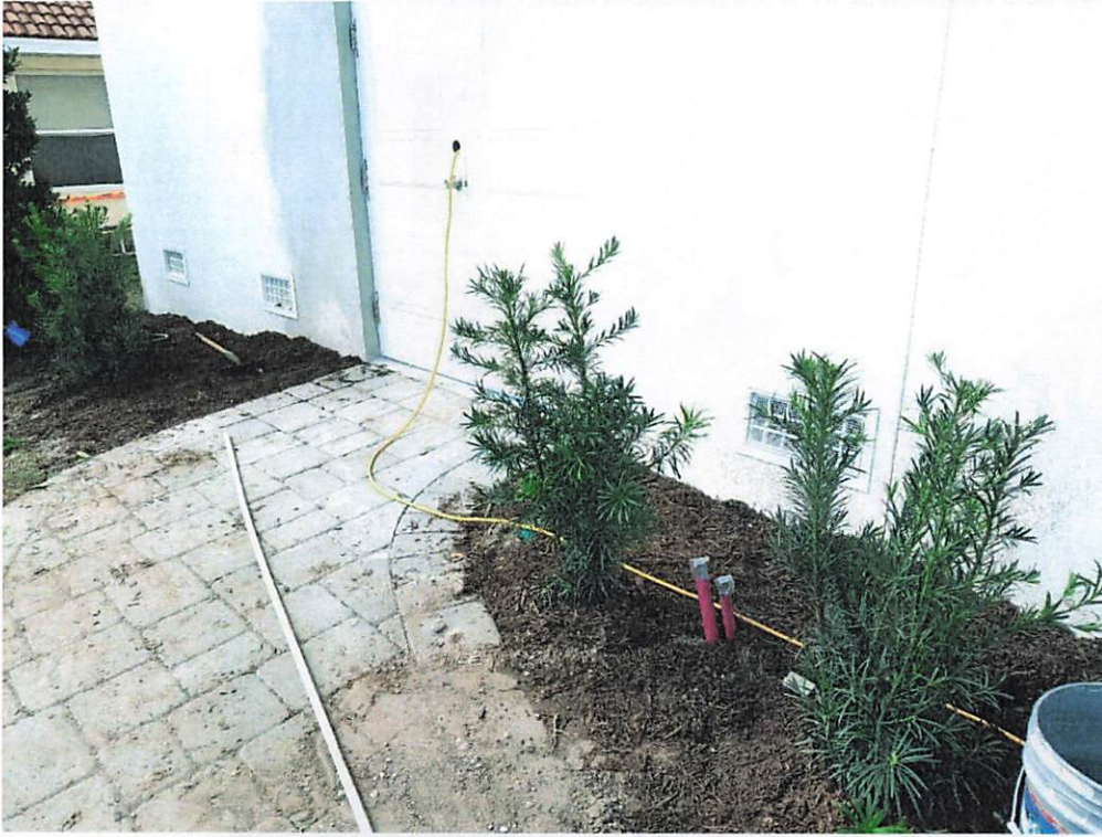
(01/26/2024) 3 Engineered Flood Flap Model #FFWF08 Rear Wall of Garage
