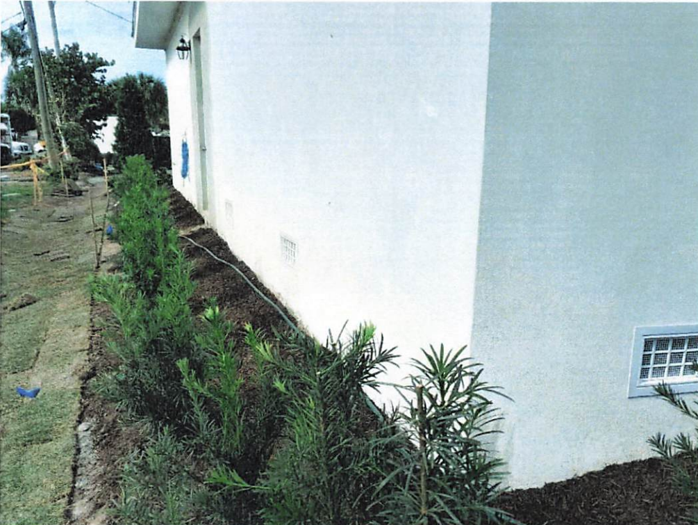
(01/26/2024) 3 Engineered Flood Flap Model #FFWF08 Right Side Wall of Garage
