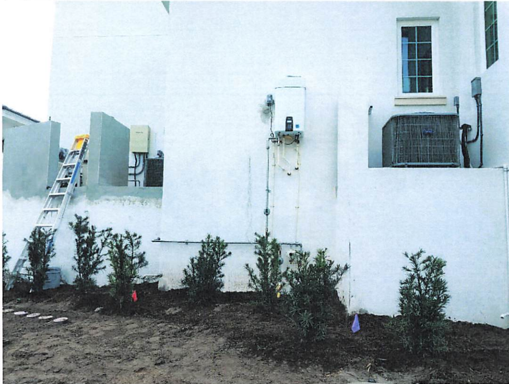
(01/26/2024) Elevated AC Units and Tankless Water Heater
