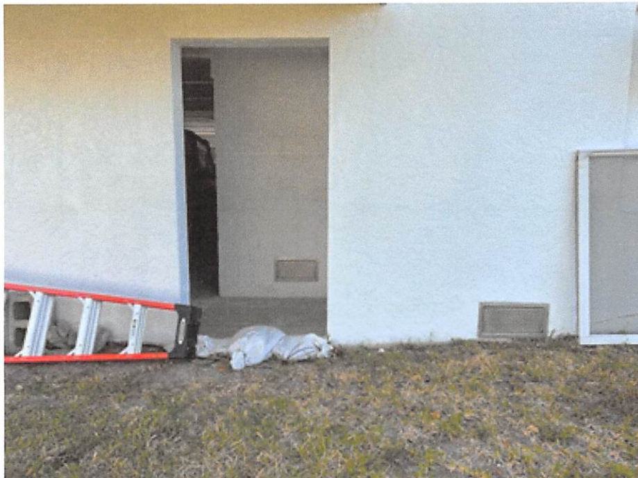
Photo Caption: 05-23-2023, Flow through, outside wall.
