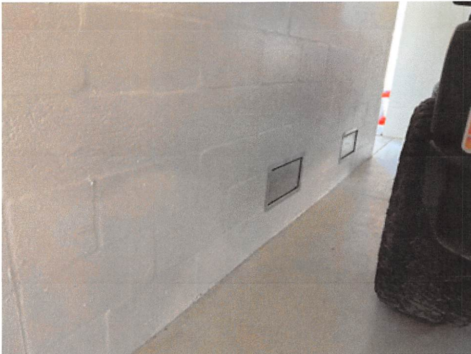
Photo Caption: 05-23-2023, FLOW THROUGH PARTIALLY ENCLOSED AREA
