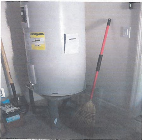
ELEVATED WATER HEATER IN GARAGE
