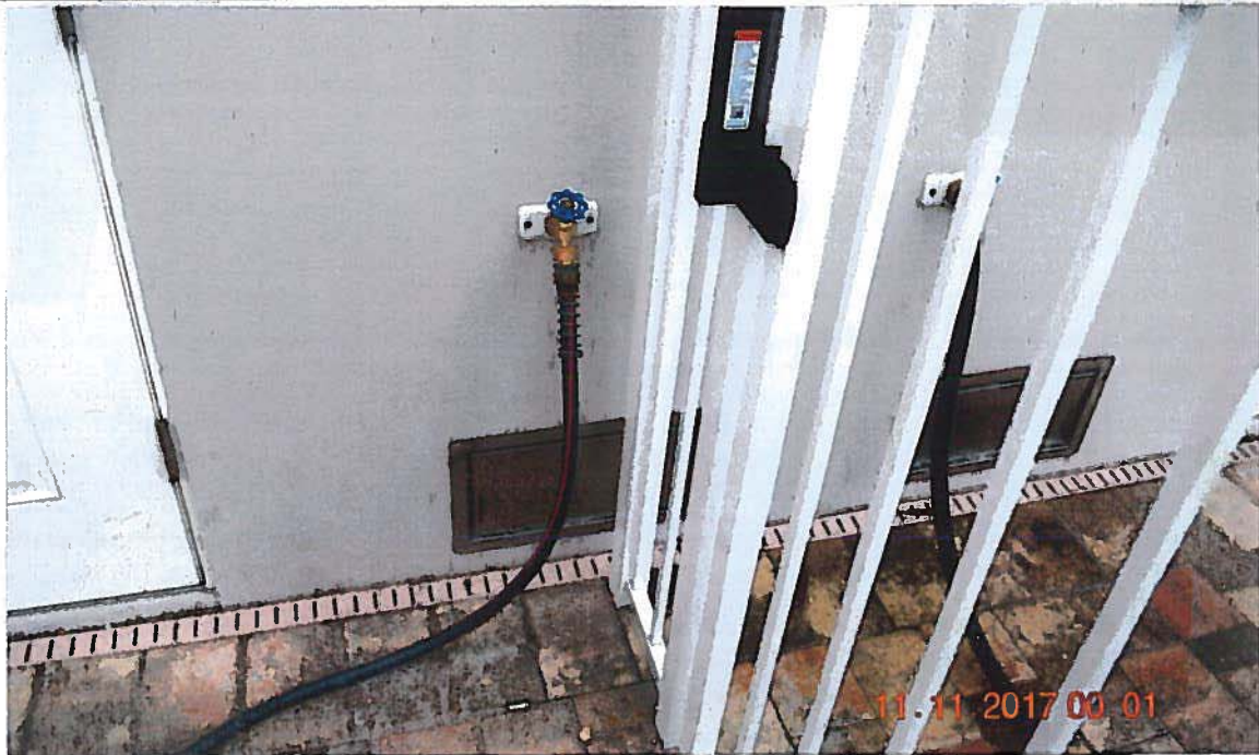
Photo Four Caption Represented Flood Vent
