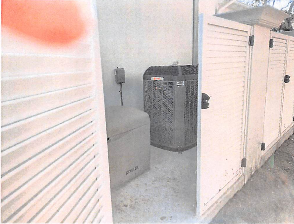
(11/02/2021) AC in Enclosure on Right Side of House/off Back of Garage
