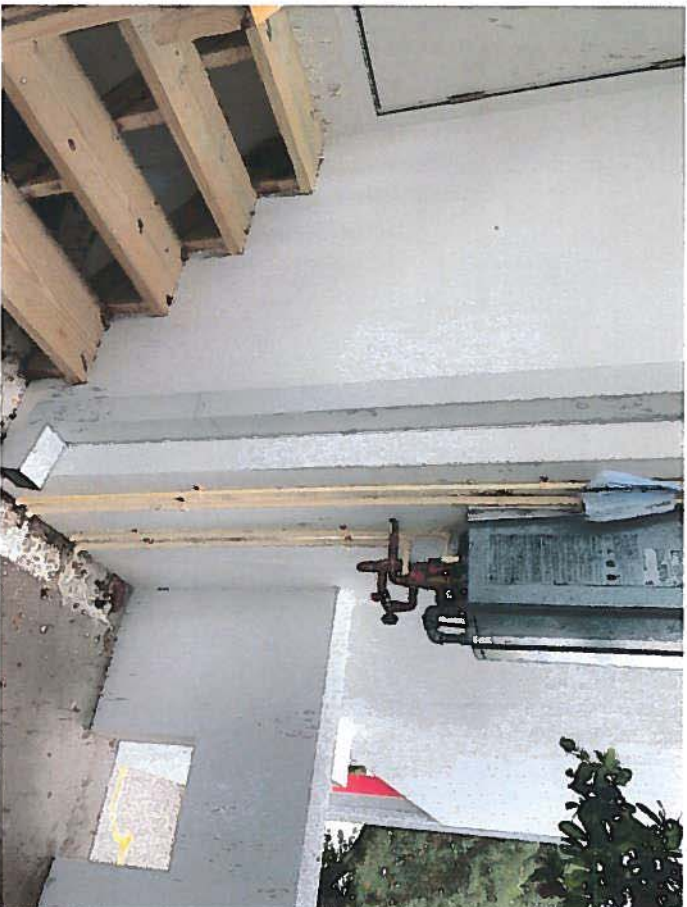
(07/10/2019) Tank Less Hot Water Heater on outside wall off 3 rd Level
