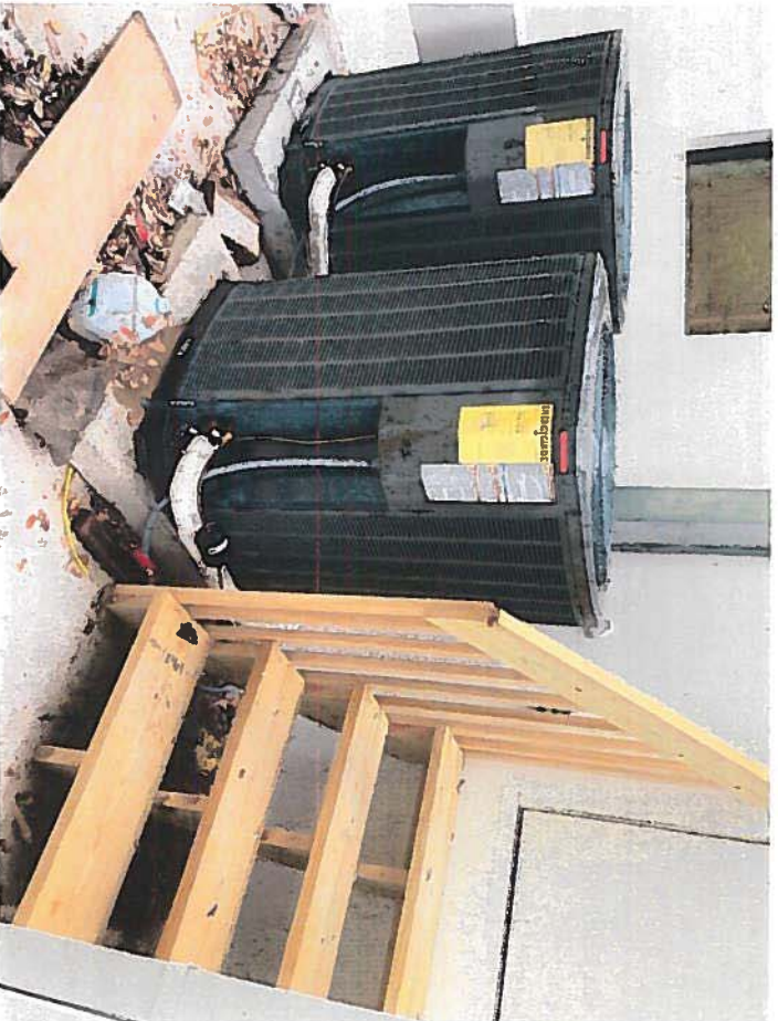
(07/10/2019) Elevated AC Units Located off 3 rd level of Structure
