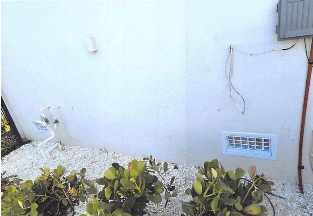
(08/08/2025) 2 Flood Flap Vents in Right Side Wall of 2 Car Garage
