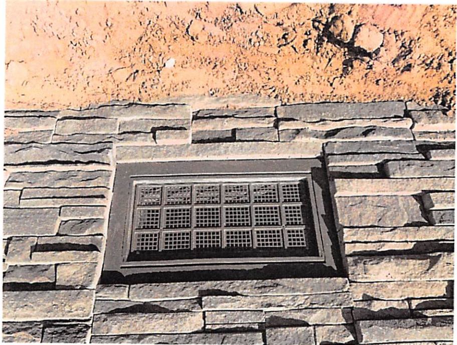
(01/28/2021) Typical Flood Vent in Garage, Storage & Foyer Exterior Walls, Flood Flap Model # FFFNF08
