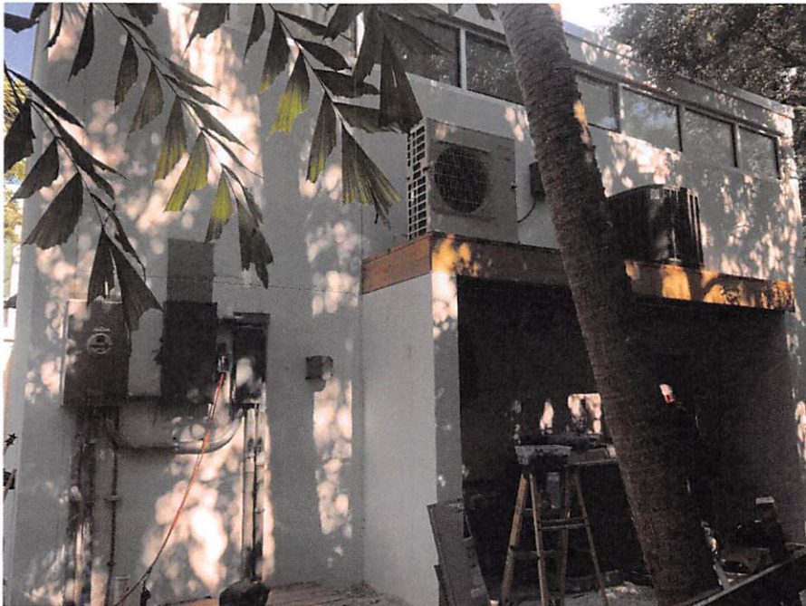
Photo Two Caption AC Condenser platform East side
