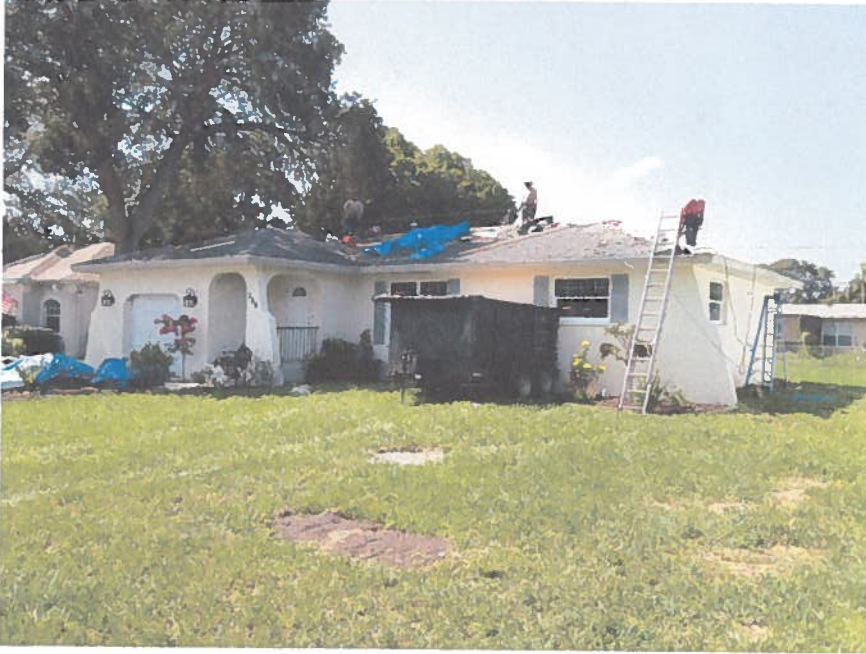
FIGURE 1: (09/15/14) FRONT & RIGHT SIDE VIEW
