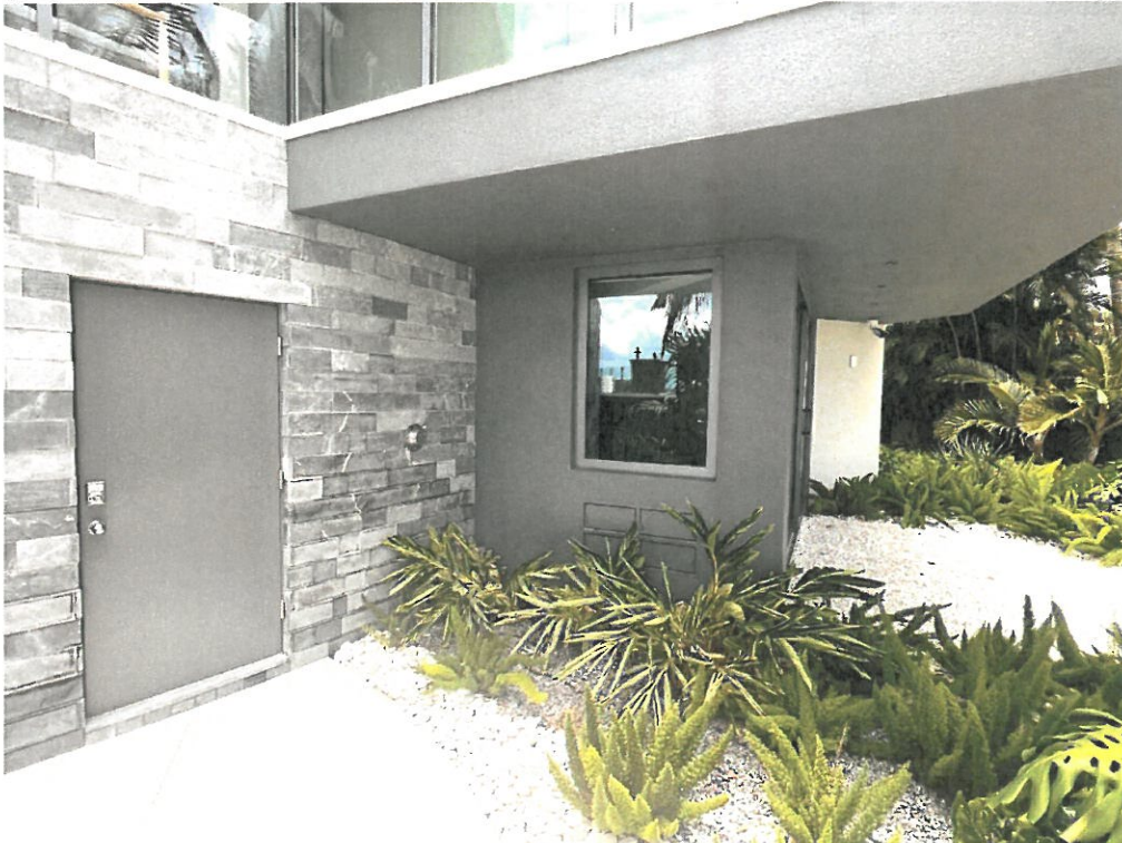
(05/24/2024) 4 Smart Vent Model #1540-520 on Rear Wall of Large Storage.
