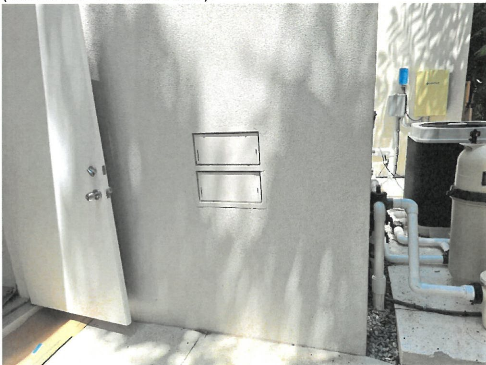
(05/24/2024) 2 Smart Vent Model #1540-520 on Right Wall of Small Storage (Within 1.0' of Finish Floor).
