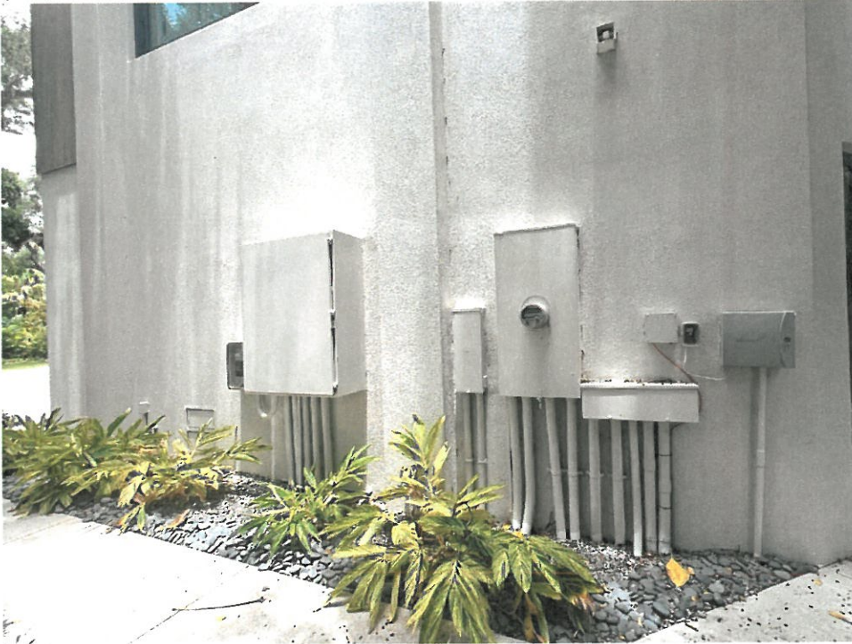
(05/24/2024) 2 Smart Vent Model #1540-520 on Right Wall of Parking Area.
