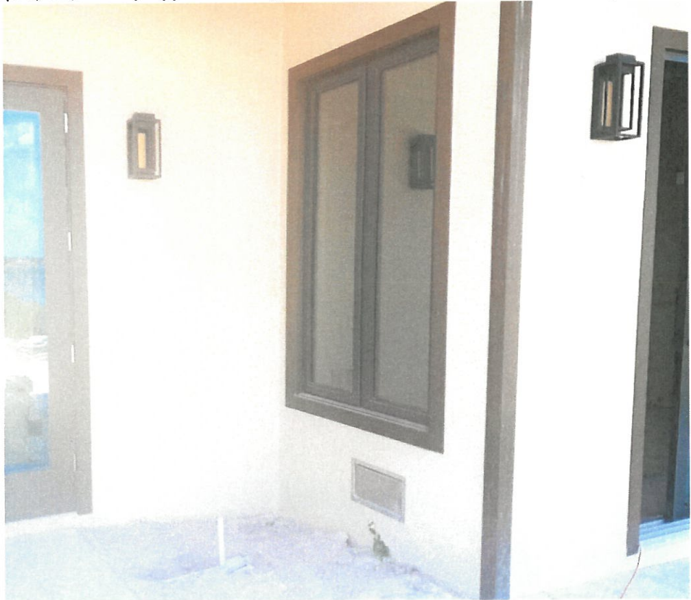
(04/09/2024) Typical 1 Engineered Smart Vent in East Wall/North Side of House
