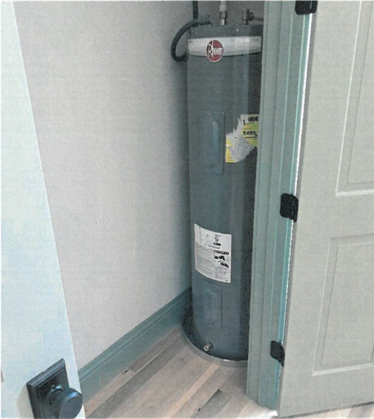
(06/14/2023) Hot Water Heater in Closet in Living Area
