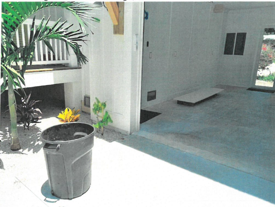
(06/14/2023) 1 Smart Vent Model #1540-570 in Exterior Wall of Entry Stairway and Storage Area from Garage, 1 Smart Vent from Room to Garage
