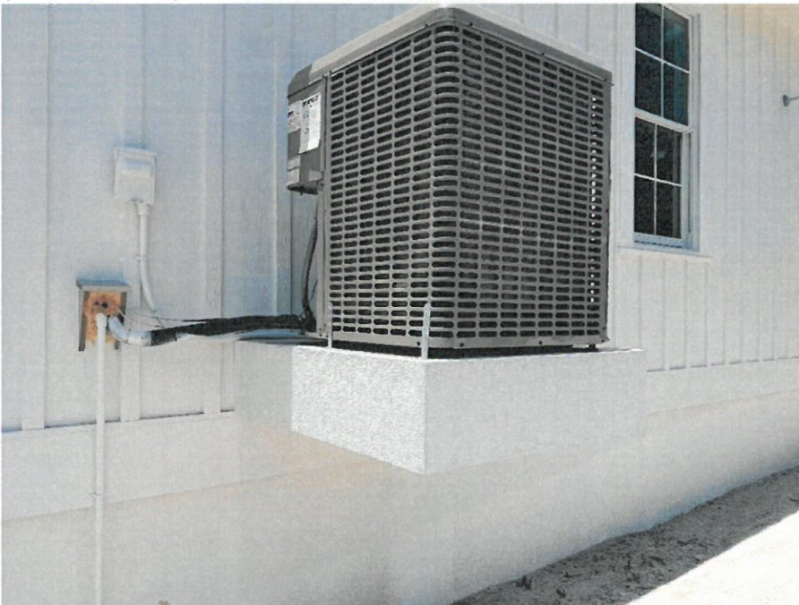
(06/14/2023) Elevated AC Unit on Outside of House
