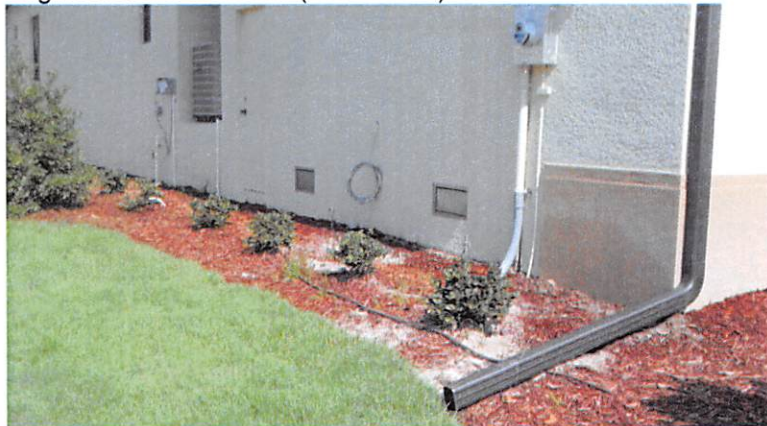
Engineered Flood Vents (South Side):
