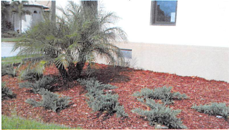
Engineered Flood Vents (North Side):
