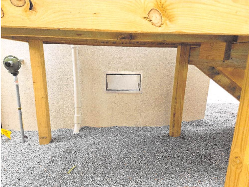
(09/04/2024) 1 Smart Vent on Left Side of Structure Under Stairs
