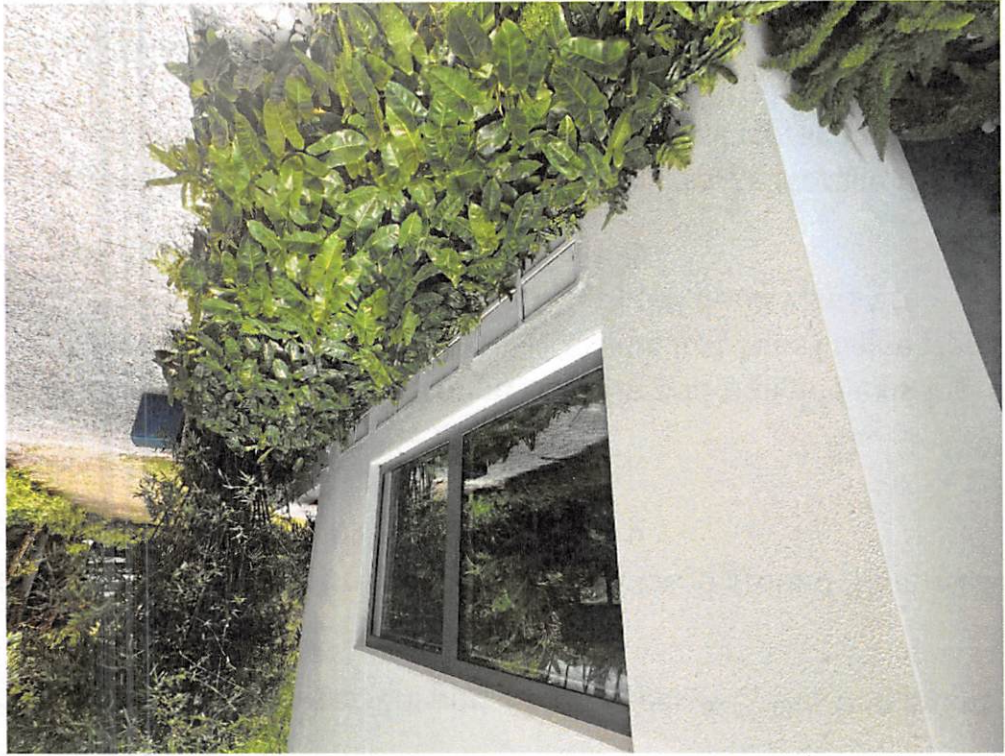
(05/24/2024) 14 Smart Vent Model #1540-520 on Left Wall of Large Storage.
