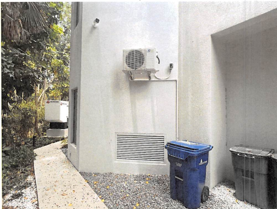
(05/24/2024) Non-Engineered Flood Vent on Rear Wall of Parking Area with Elevated Wall Mounted AC Unit, Elevation = 14.1.
