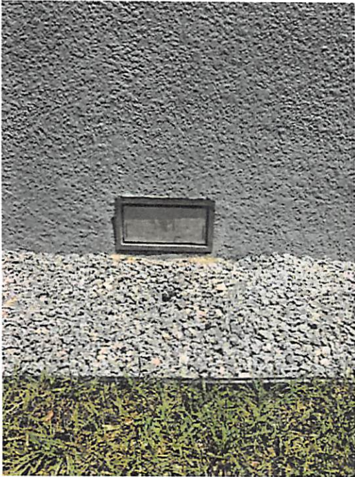
SMART VENT INSTALLED & VENT TAG 4/25/24
