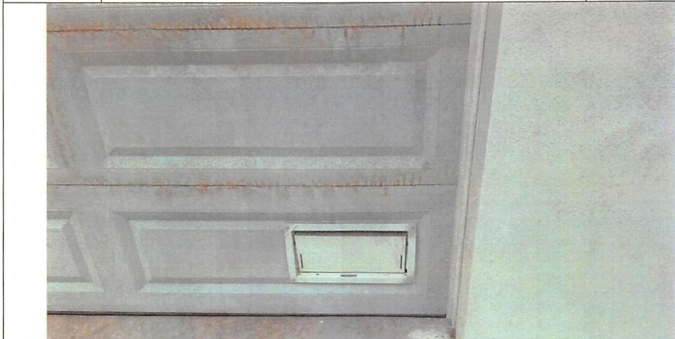
Photo 6 Caption Smart Vent Detail JOB# 20-1466 Date Taken 5/15/23
