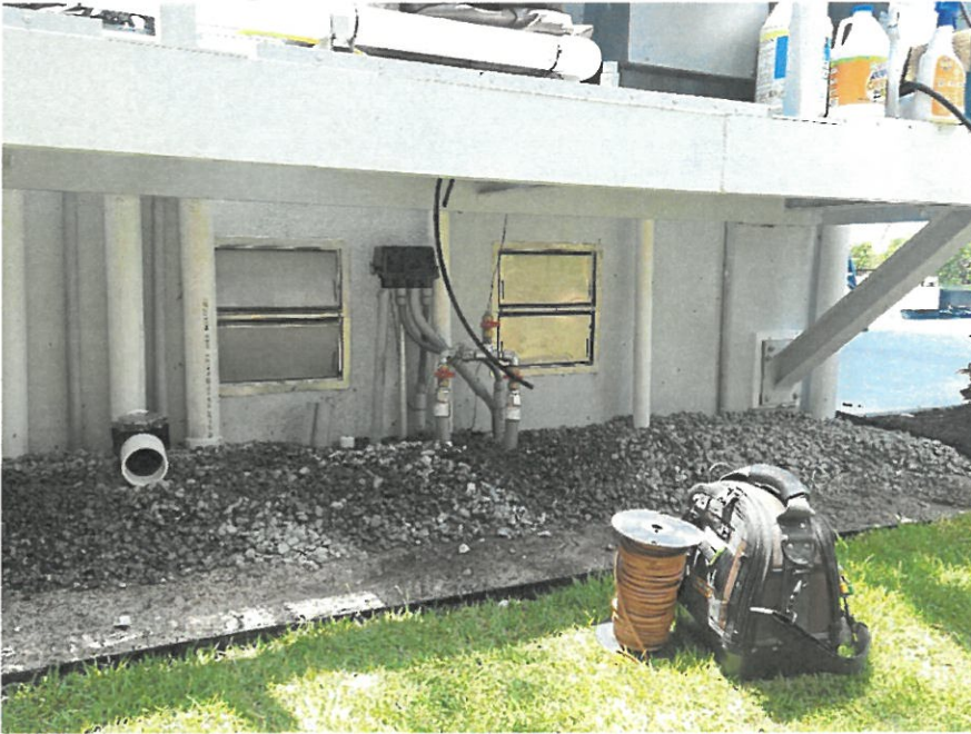
(05/21/2026) Typical Double Smart Vents under Elevated Pool Equipment Platform on Right Side Wall on rear of Structure.
