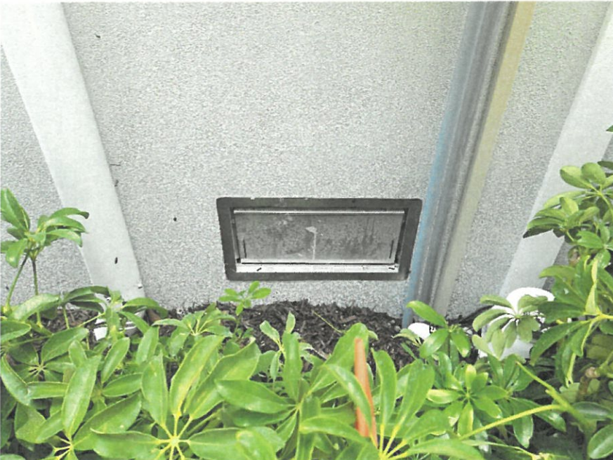
(05/21/2026) Typical Single Smart Vent on Front, Left & Right Side Walls of Structure.
