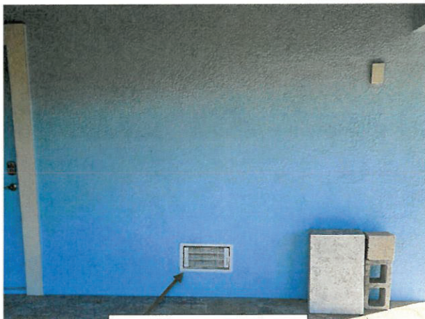
Garage A - Vent #5
