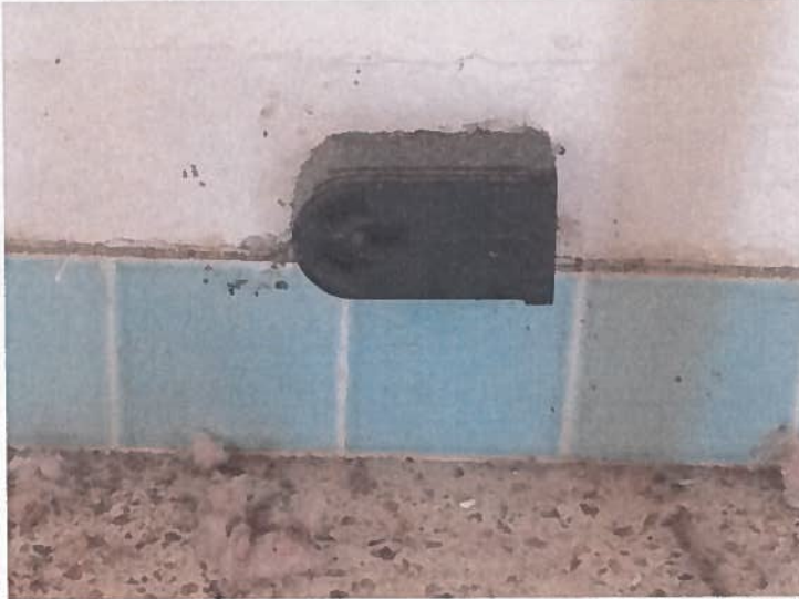
LOWEST EQUIPMENT SERVICING THE BUILDING IS A STOVE ELECTRICAL OUTLET. 08/19/2015
