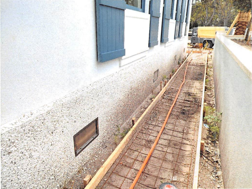
(04/24/2024) North Garage Wall with 4 Engineered Smart Vents.
