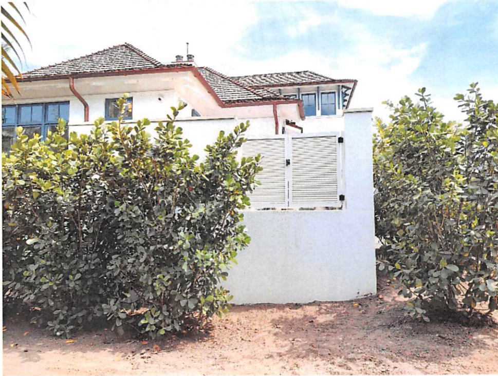
(04/24/2024) Lowest Equipment, Top of AC Enclosed Platform =11.0', Located on Left/North Side of House.
