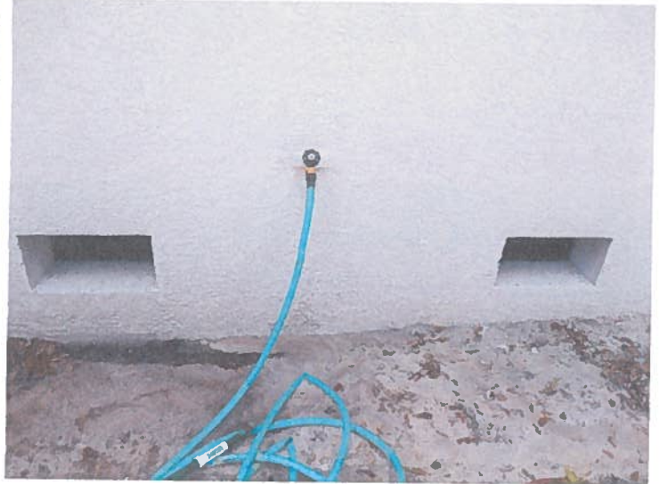
FIGURE 5: (04/20/15) FLOW THRU VENT
