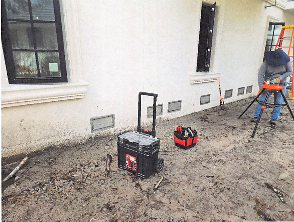
(10/01/2024) Portion of Right Side Wall at Front, 7 Smart Vents
