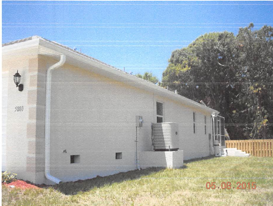
Right Side View Elevated A/C Pad & Flood Vents
