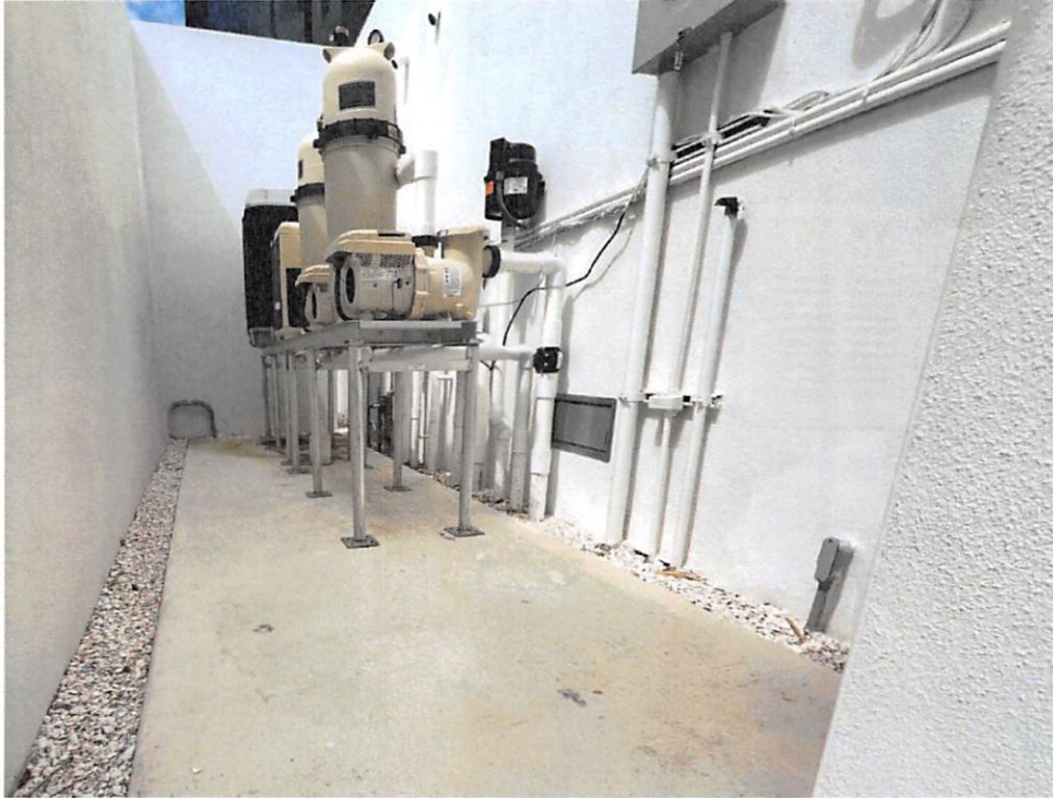
(04/18/2024) 1 Smart Vent in Parking Area South Wall in Pool Equipment Area
