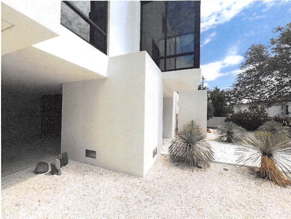
(04/18/2024) 2 Smart Vents in Storage Area Walls
