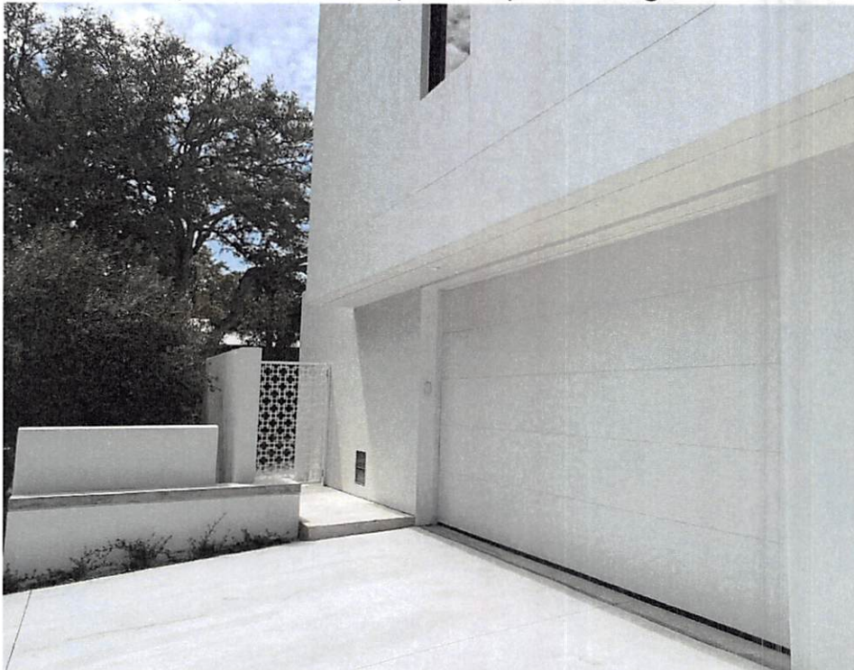
(04/18/2024) 2 Smart Vents (stacked) in Parking Area East Wall
