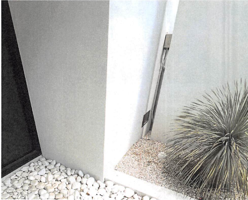
(04/18/2024) 1 Smart Vent in Parking Area South Wall
