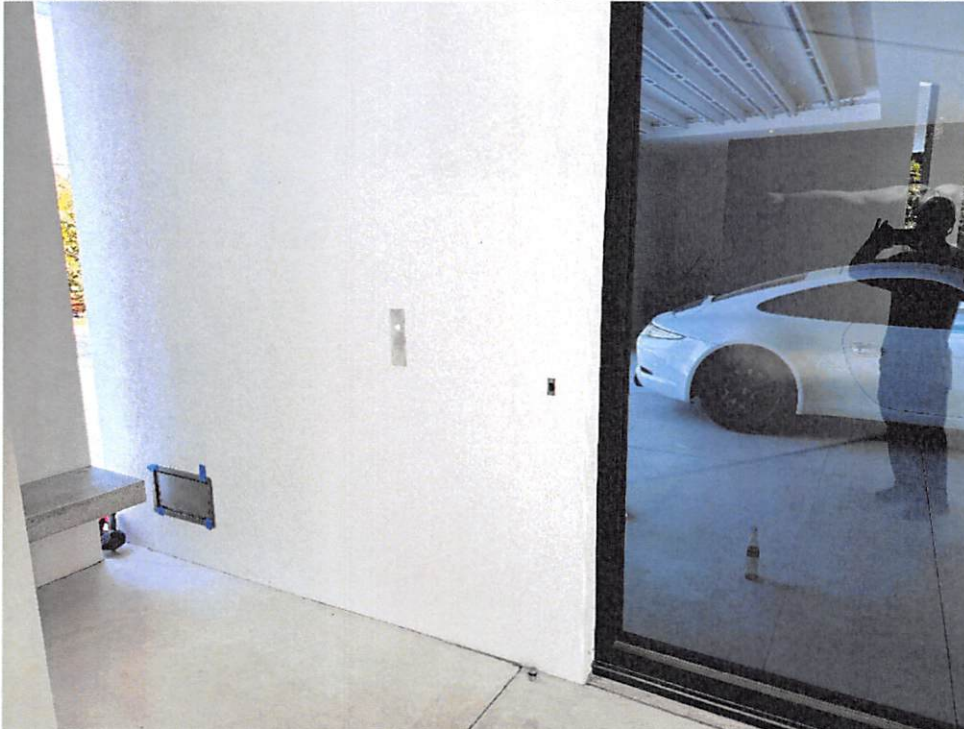
(05/21/2024) 1 Smart Vent in Parking Area North Wall Added on This Date
