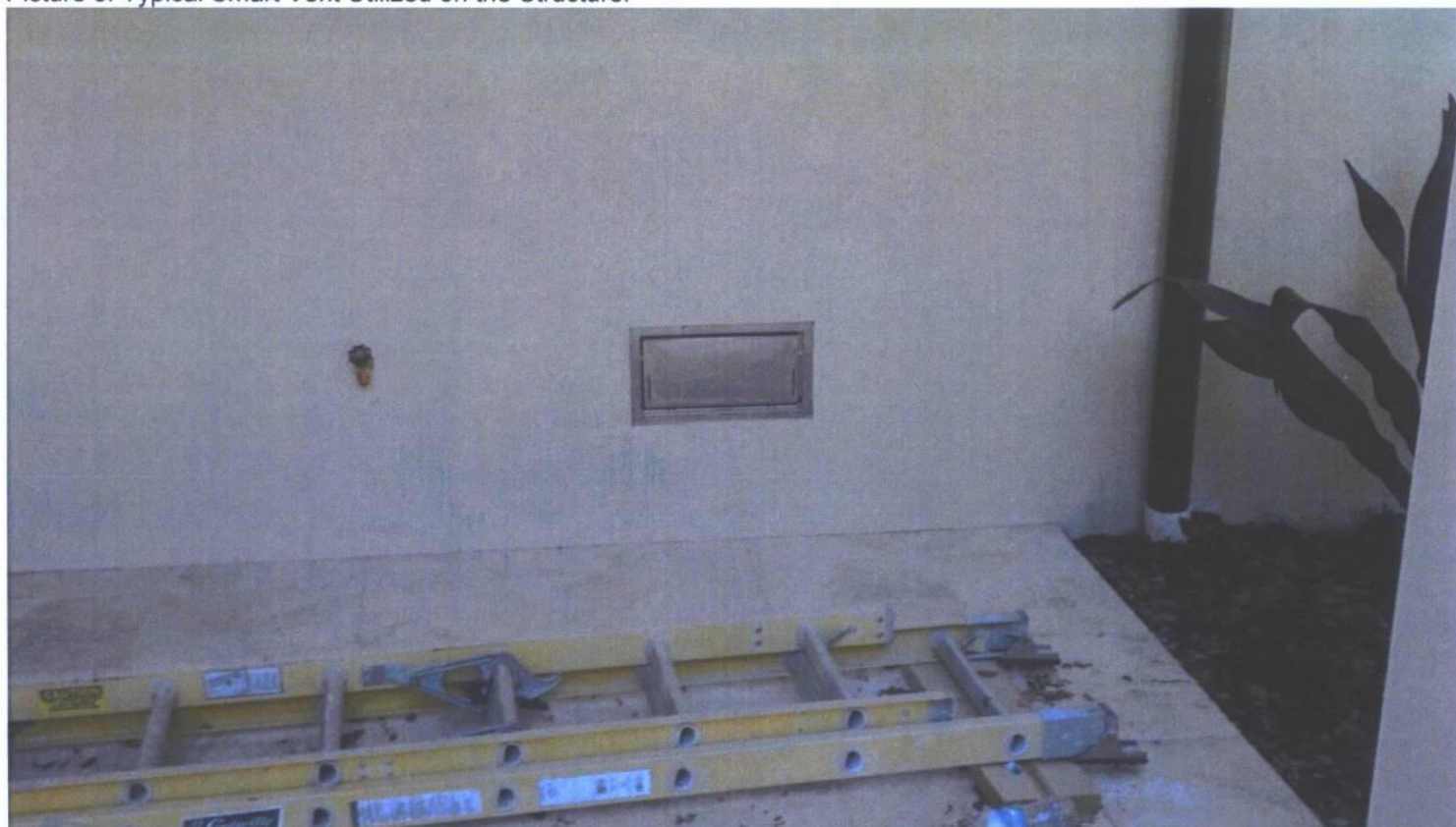
Picture of Typical Smart Vent Utilized on the Structure:
