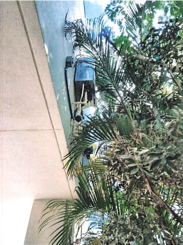
(12/21/2023) Raised Tankless Water Heater = 18.7', Located on Outside Wall.
