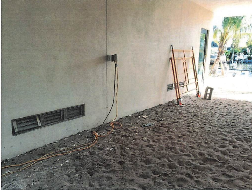
(12/21/2023) 6 Smart Vents Model #1540-510 in Garage 1, Right Side Wall
