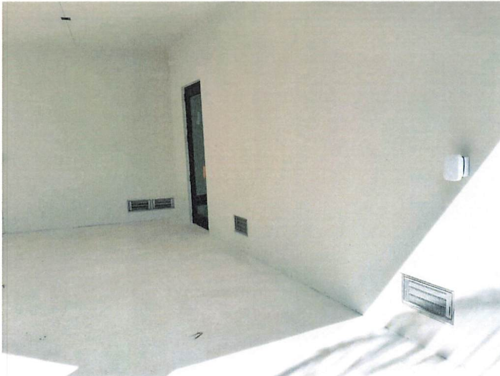
(12/05/2023) 2 Smart Vents Model #1540-510 in Garage 1, Rear Wall & 2 Smart Vents Model #1540-510 in Right Side Wall of Storage/Crawl Space Area
