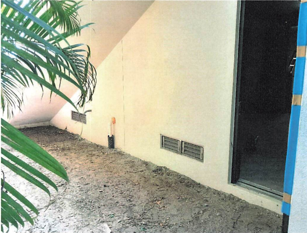
(12/21/2023) 4 Smart Vents Model #1540-510 in Storage/Crawl Space Area
