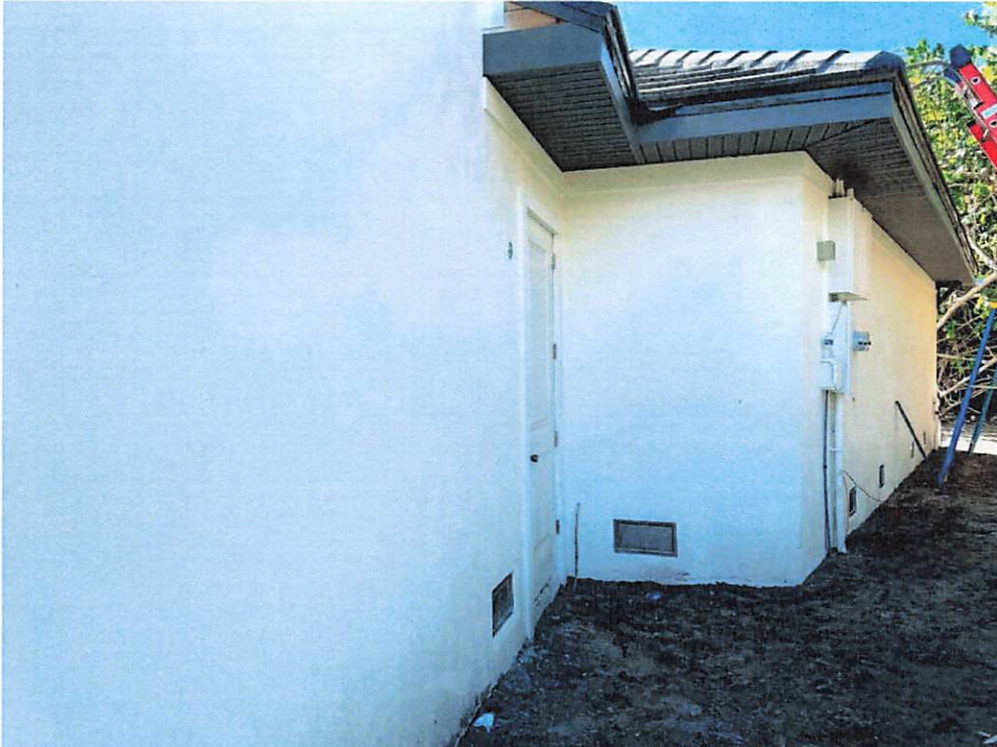
(11/20/2023) 6 Smart Vents Model #1540-520 in Garage Walls
