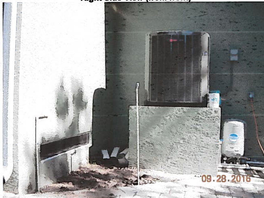
Elevated A/C Pad
