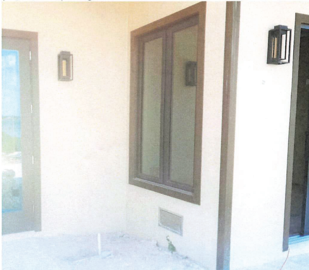
(04/09/2024) 1 Engineered Smart Vent in East Wall/North Side of House
