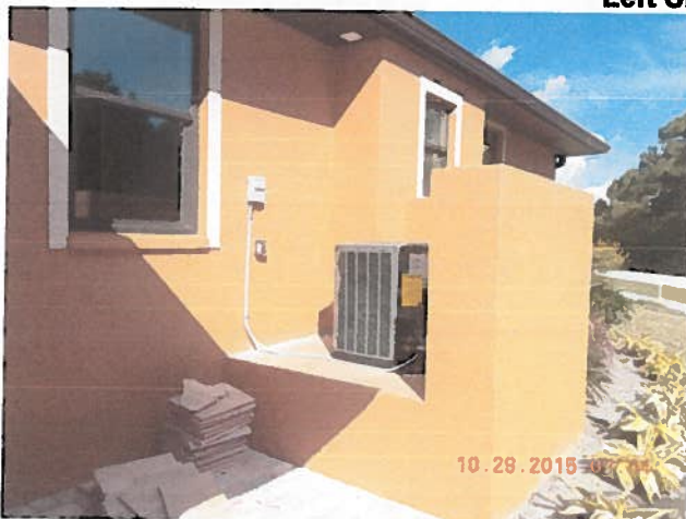
Elevated A/C Pad
