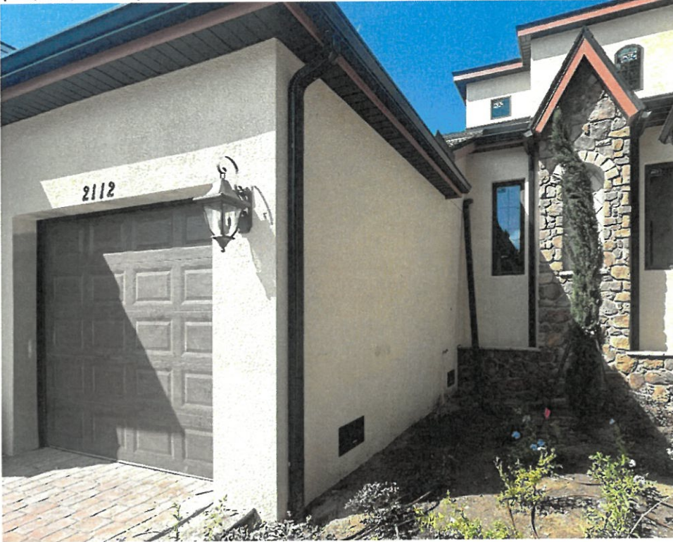
(05/27/2025) 2 Flood Vents on Right Side Wall of Garage
