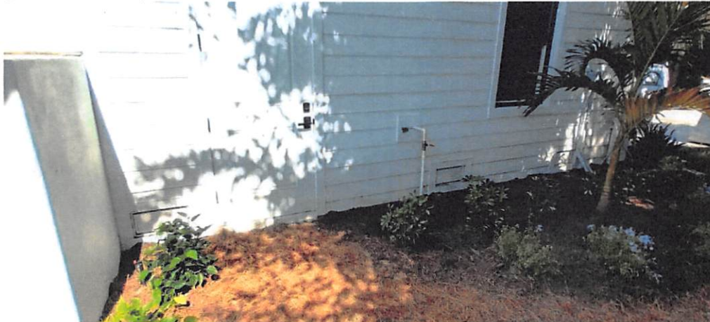
(10/27/2023) 3 Smart Vents Model#1540-510 in Left Wall of Garage.
