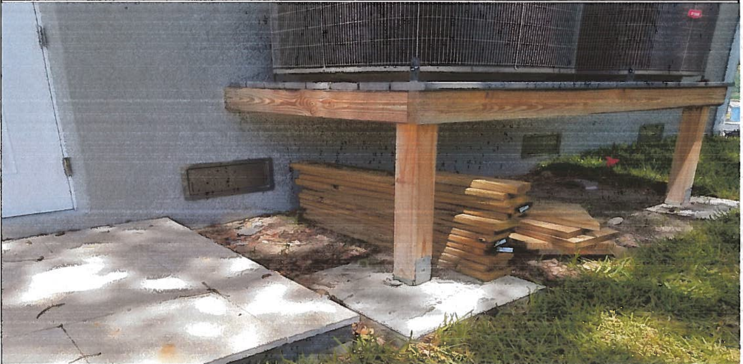
Photo One Caption 1614 Anchorage Street - Vent Photos
